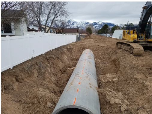
Davis and Weber Counties Canal Company's Small Piping and Hydro Project in Utah, which was an FY 2018 Water and Energy Efficiency Grant project. Photo courtesy of Davis and Weber Counties Canal Company.
